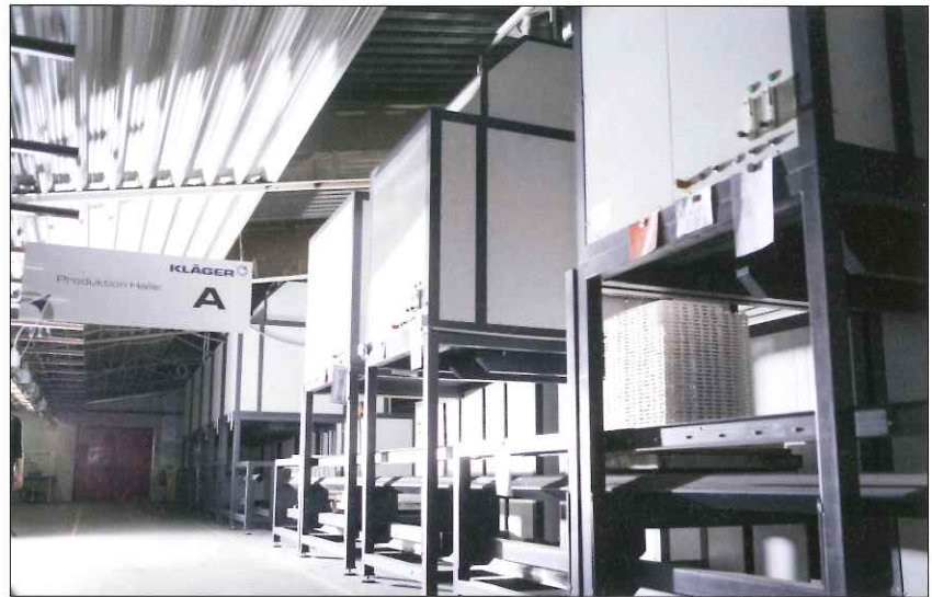
Fig. 6 Debinding and sintering equipment
